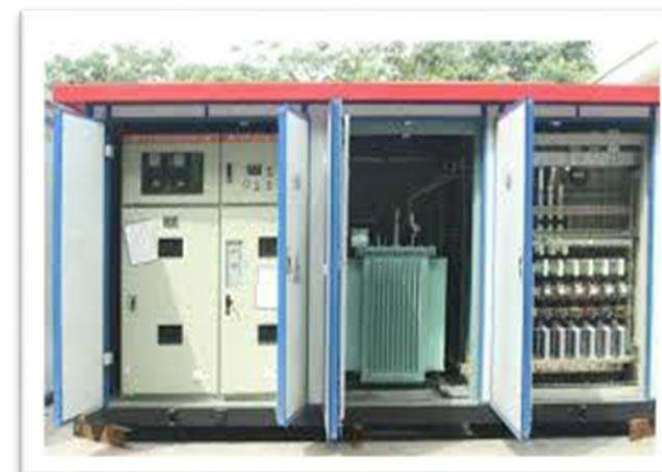
Compact Sub station
