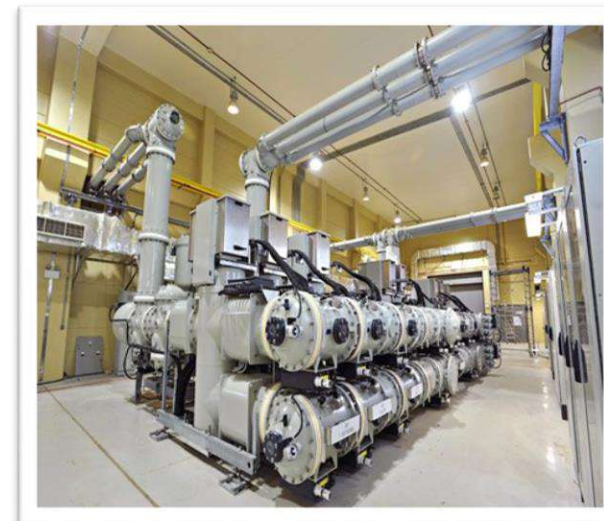
GIS Sub station
